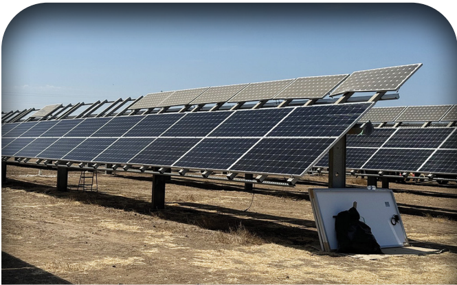
Figure 7. For PV1, spot-welded bolts complicated removal and replacement of legacy c-Si modules. (Credit: SSJID)
