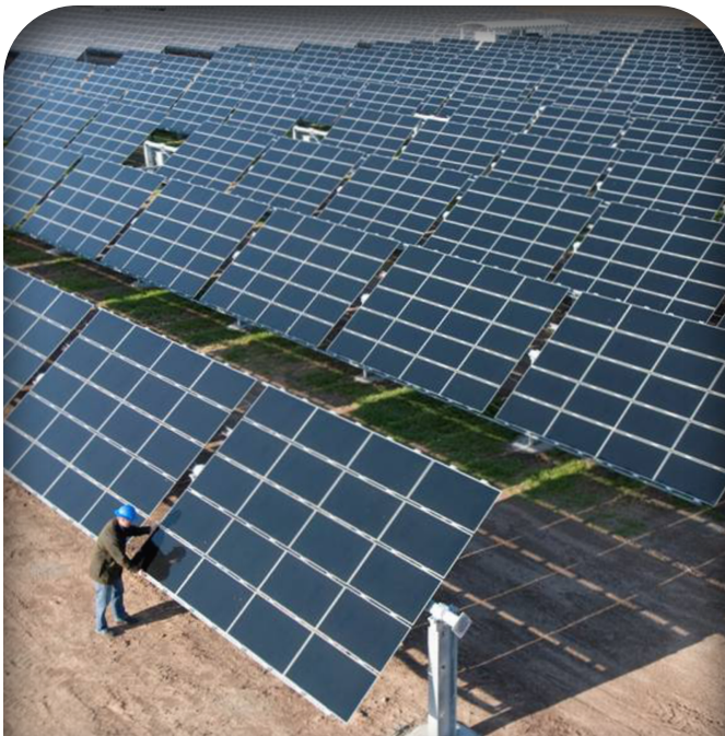
Figure 3. After a productive first decade, the solar farm's degraded performance created needs for more proactive asset management. (Credit: SSJID)
