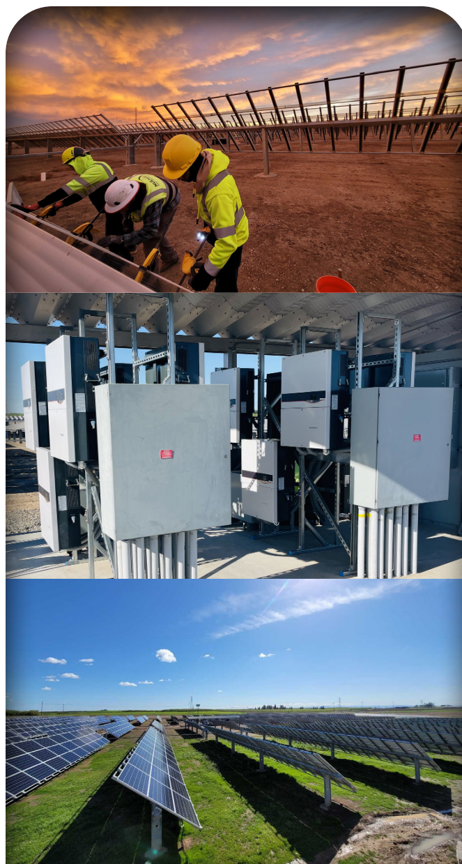
Figure 12. Reusing underground conduit (top) to supply string inverters and other equipment deployed on the existing concrete pad (middle) were key elements to successful redevelopment (bottom). (Credit: NuLife Power Services)
